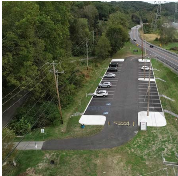
Parking is a critical trailhead component for most trails.
